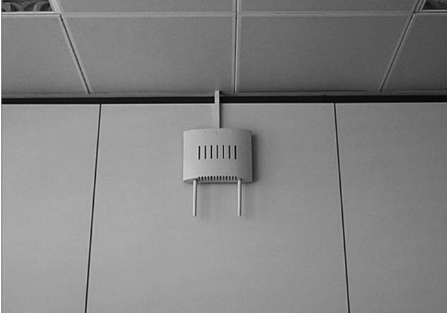
Figure 18: Access point for DECT systems
